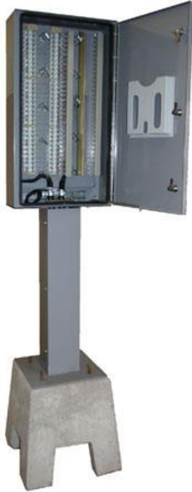
Passcomm Box On Post
